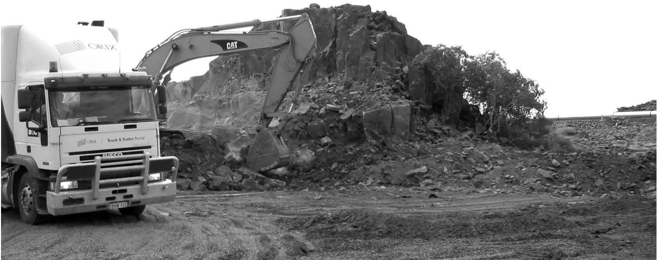
Figure 2. Destruction of rock art site for road fill, on 30 May 2006, near Dampier Port.
